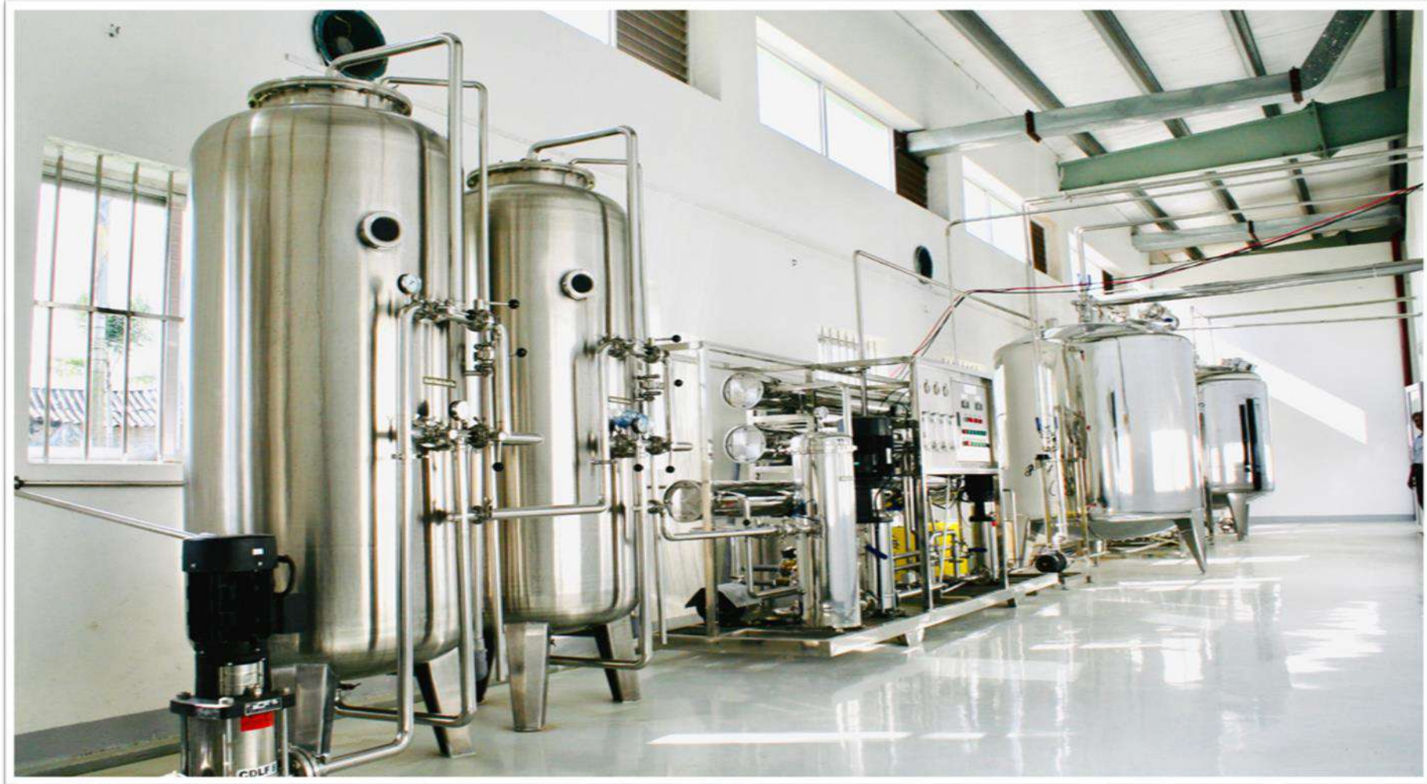
Reverse Osmosis (RO) and Distilled Water Treatment Systems
